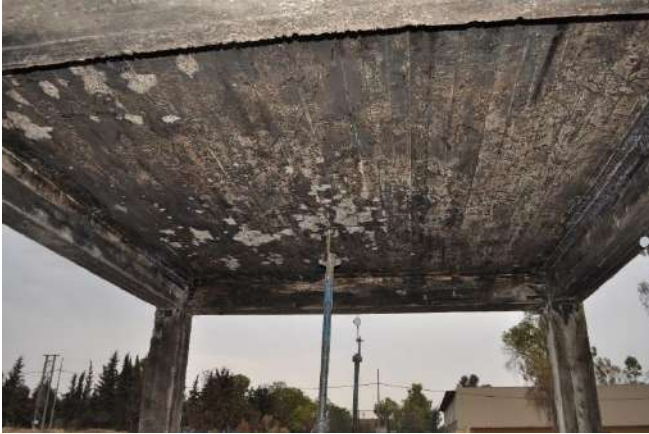
Figure 16: Spalling and change color occurred in slab
